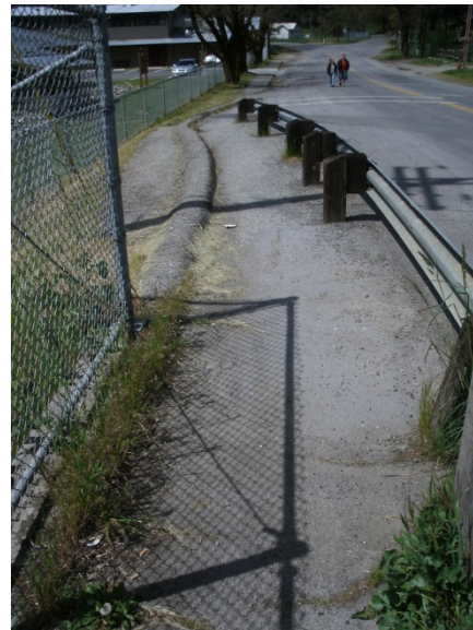
Figure 3 – Non-ADA compliant pedestrian access at west end
