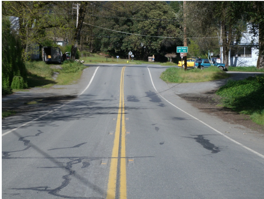
Figure 2 – Roadway dip, approaching from west
