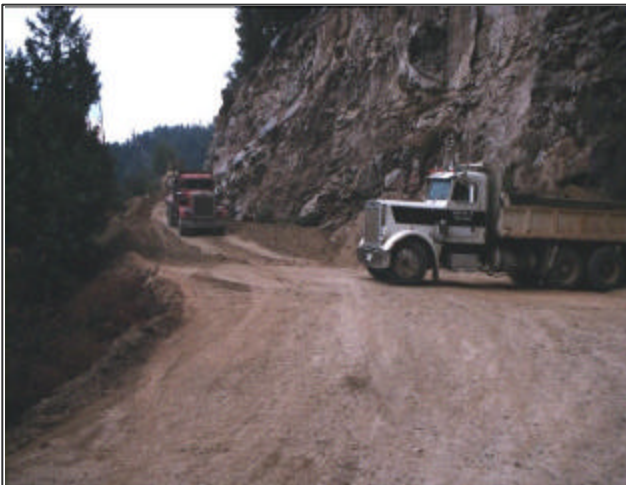
Trucks disposing of fill from RX10 into RR2 near photo point on right.
